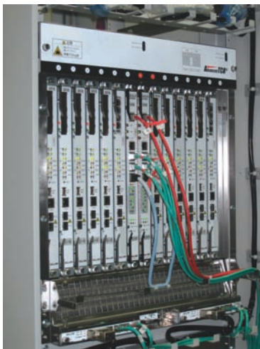
Fig. 5. Example of server shelves.
