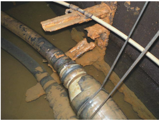
Fig. 1. Cable bearer broken as a result of corrosion.
