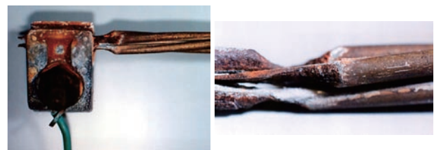
Fig. 5. Fractured AW messenger wire.
