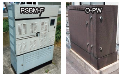
O-PW: Outdoor Cabinet with Power RSBM-F: Remote SuBscriber Module-Feeder
