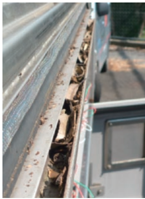
Fig. 4. Clogged drainage duct.
