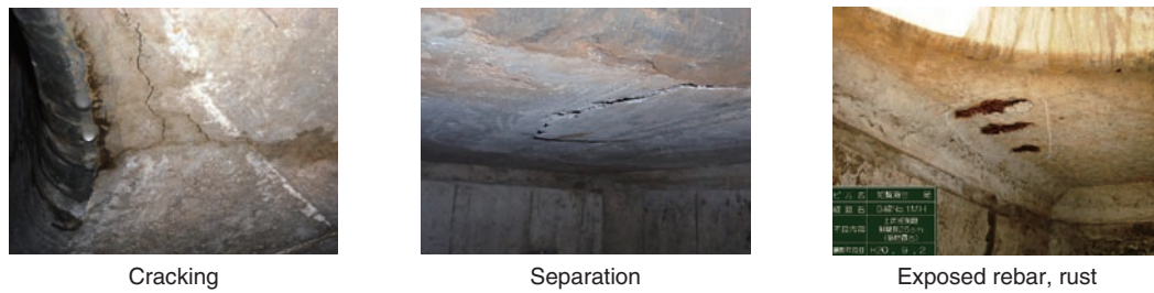
Fig. 3. Types of manhole degradation.
