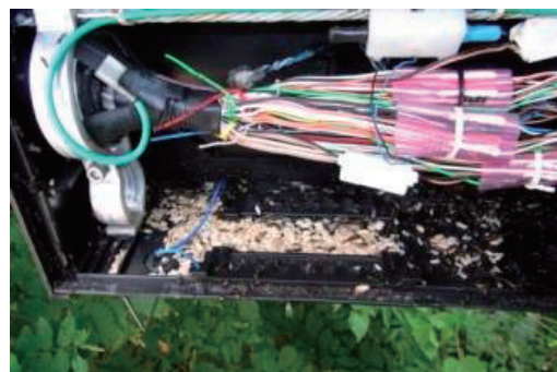
Photo 4. Interior of metal terminal box in which core-wire insulation is broken.
