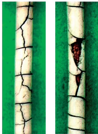
Fig. 1. Deterioration of insulating coating of electrical wires.
